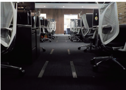
Oizumi Studio main building air-conditioning floor vents
